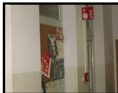
Fig. 25: Manual fire alarm system
