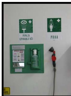
Fig. 13: Eye wash and emergency shower
