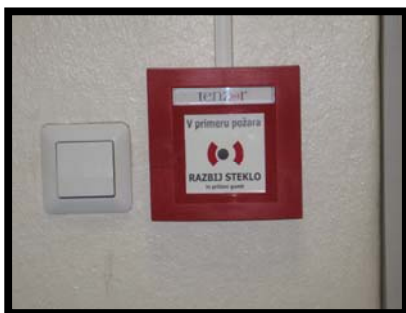
Fig. 24: Manual fire alarm system
