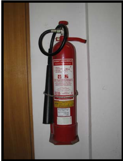
Fig. 18: Manual fire extinguisher
