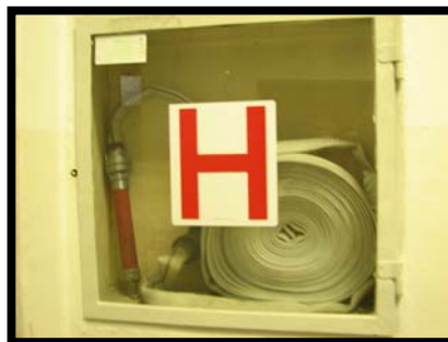
Fig. 20: Indoor fire hydrant
