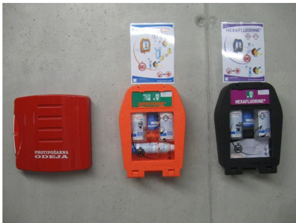
Image 13: Wash stations in case of corrosive substance spillage Defibrillator
