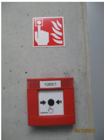
Image 19: Manual fire alarms
