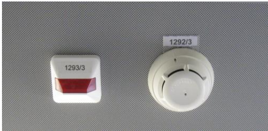
Image 18: Automatic fire alarm (right) and alarm indicator (left)
