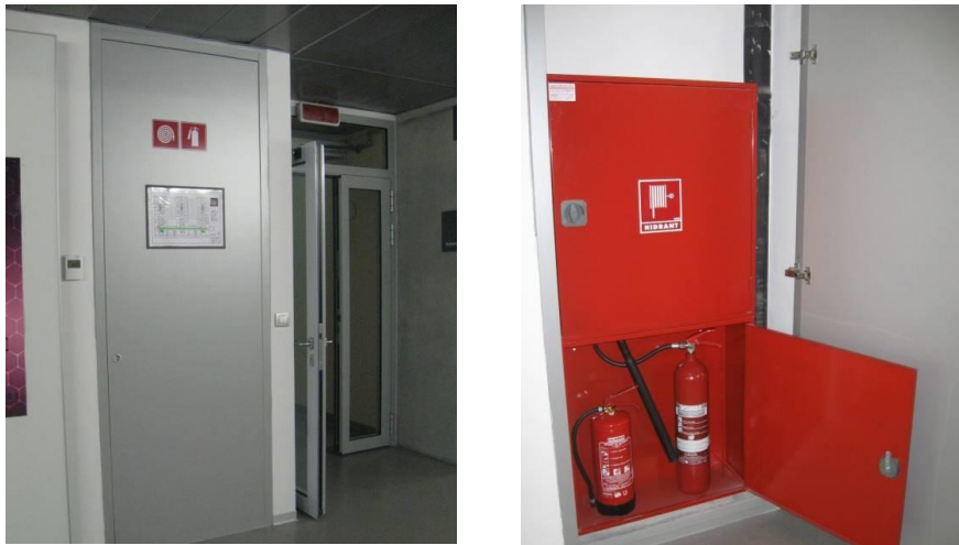
Image 23: A cabinet containing a hydrant and the two fire extinguishers.
