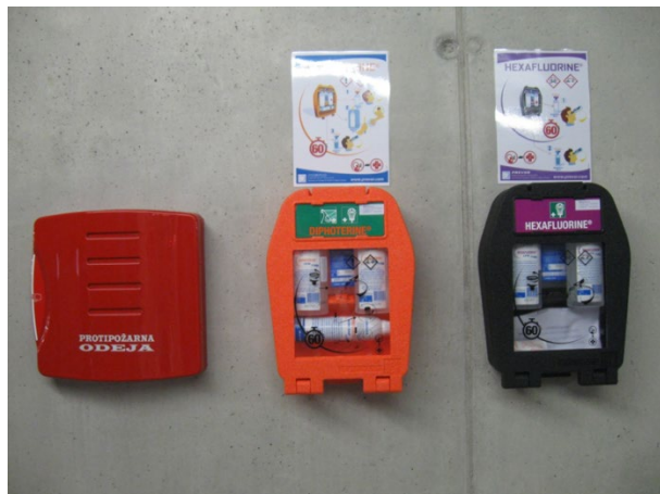
Image 15: Wash stations in case of corrosive substance spillage
