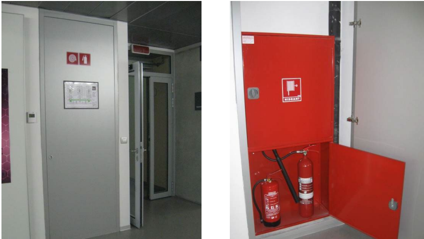
Image 26: A cabinet containing a hydrant and the two fire extinguishers.
