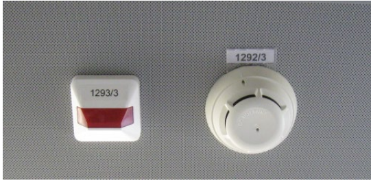
Image 21: Automatic fire alarm (right) and alarm indicator (left)
