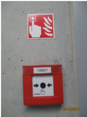
Image 22: Manual fire alarms
